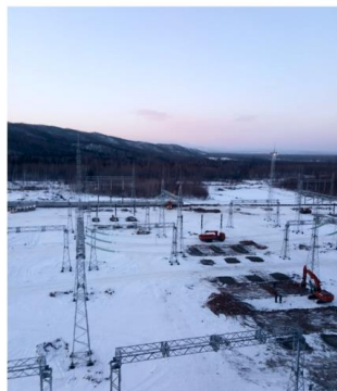
Switchgear bushing portals
